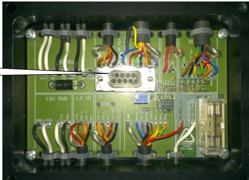
FCC (FES connecting circuit) view with cover removed.
